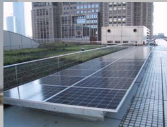
PV generators on the top of metropolitan assembly building
